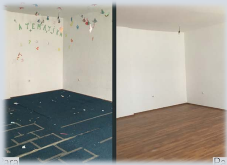
Photo 7. One of the photos taken during the renovation of “Roma Mahalla” learning center in Mitrovica.
